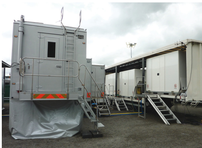
The GPPU unit (left) and three containers that house the flyaway units loaded on the flat bed (right)
